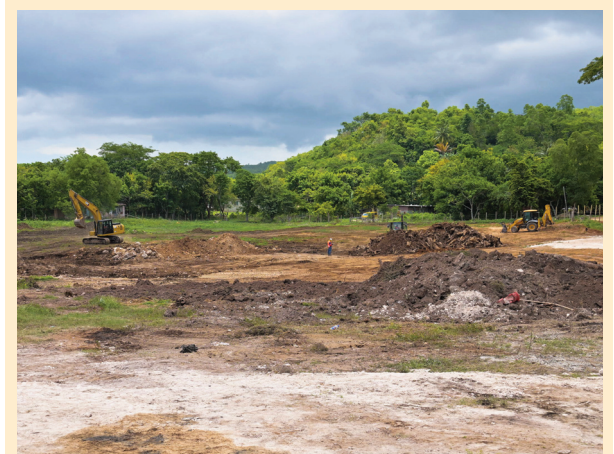
Excavation work being carried out at the Rio Cobre Water Treatment Plant project site in Content, St. Catherine, ahead of the start of construction.
