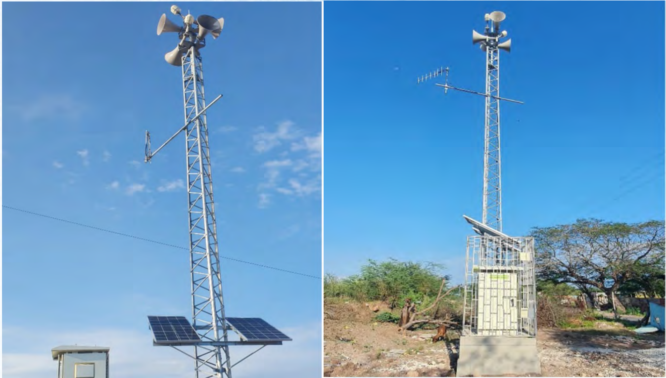
Early Warning siren towers
