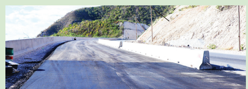
A section of the Southern Coastal Highway Improvement Project (SCHIP) in Grants Pen, St. Thomas.
