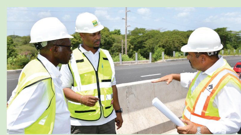
Minister without Portfolio in the Ministry of Economic Growth and Job Creation, Hon. Everaldo Warmington (left), and Director, National Road Operating and Constructing Company Limited (NROCC), Steven Edwards, listen as Resident Engineer, SJE Consultants Limited, Raul Brito, explains aspects of work undertaken on the May Pen to Williamsfield (Phase A) leg of the Southern Coastal Highway Improvement Project (SCHIP), during a recent tour.
