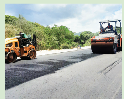
Paving works are in progress on the St. Thomas leg of the Southern Coastal Highway Improvement Project (SCHIP).
