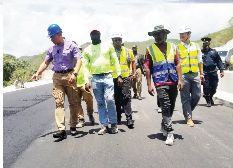
Prime Minister the Most Hon. Andrew Holness (left) points to something of interest, while walking along a paved section of the Grants Pen roadway during a tour of the St. Thomas leg of the Southern Coastal Highway Improvement Project (SCHIP) recently. He is accompanied by personnel from the National Works Agency (NWA) and China Harbour Engineering Company Limited (CHEC).
