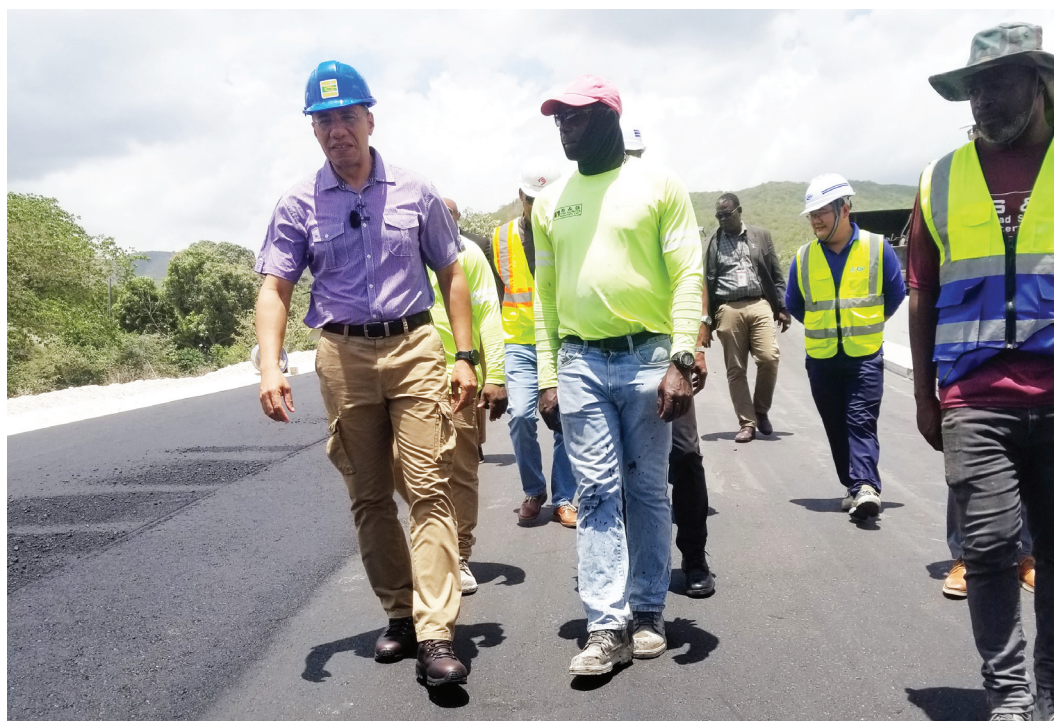
Prime Minister the Most Hon. Andrew Holness (left) walks along a paved section of the Grants Pen roadway during a tour of the St. Thomas leg of the Southern Coastal Highway Improvement Project (SCHIP) on April 13. He is accompanied by personnel from the National Works Agency (NWA) and China Harbour Engineering Company Limited (CHEC).
