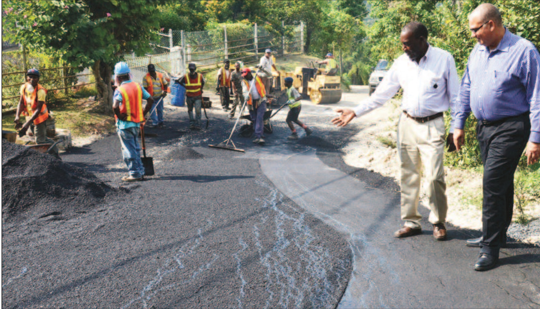
State Minister for Transport, Works and Housing, Hon. Richard Azan (right), is shown repairs being carried out on the Brandon Hill main road in West Rural St. Andrew under the Jamaica Emergency Employment Programme (JEEP) by Director of Major Projects at the National Works Agency (NWA), O'Reilly Henry. The road was one of several in the constituency which was repaired at a cost of $280 million.
