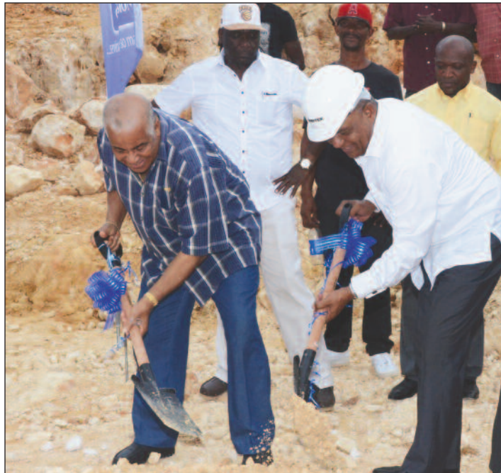
Minister of Water, Land, Environment and Climate Change, Hon. Robert Pickersgill (left), and Member of Parliament for North Clarendon, Hon. Horace Dalley, break ground for the construction of a $35.7 million water storage facility at Mason River.
